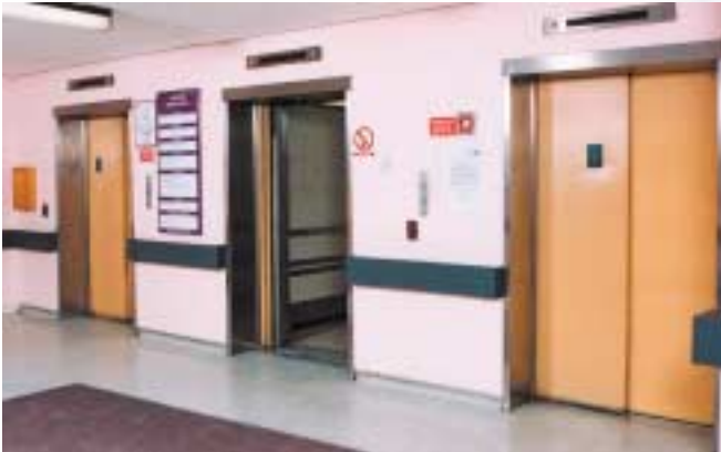
Triplex bed passenger lifts prior to modernisation
